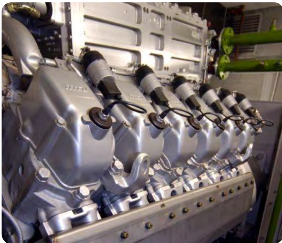
1.6 MW CHP at Loughborough University from ENER-G
