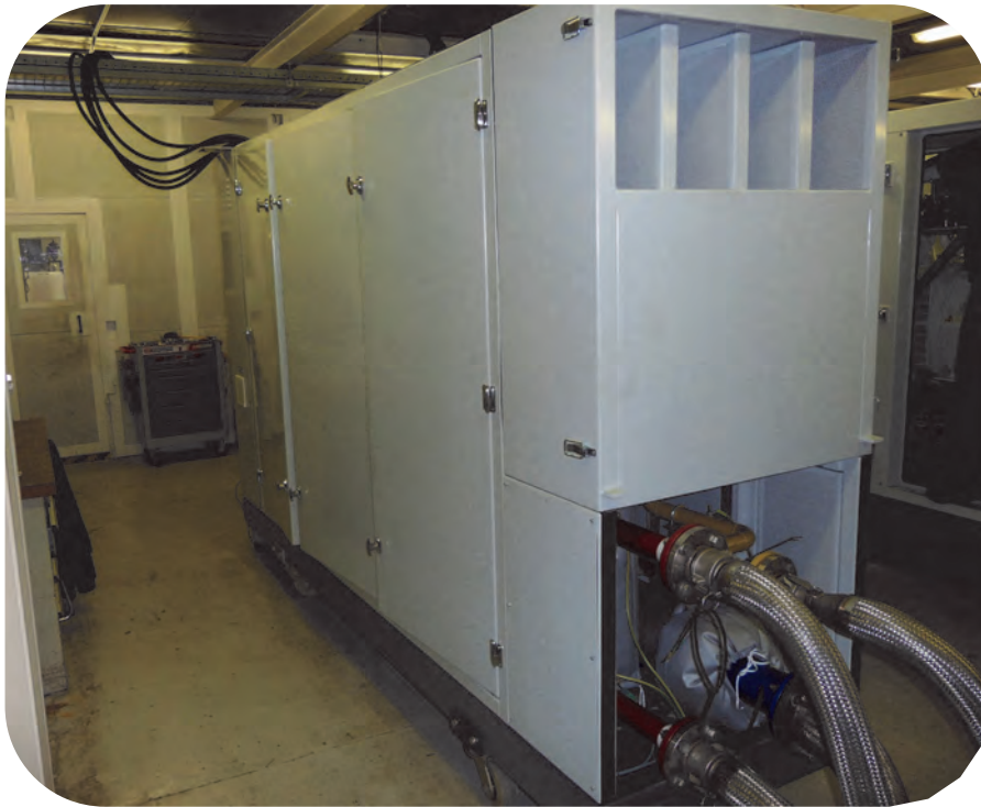
Queen Elizabeth school ENER-G 70kW CHP Unit
