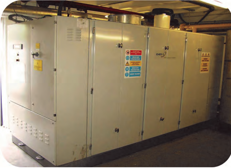
Hampton school ENER-G 150kW CHP Unit
